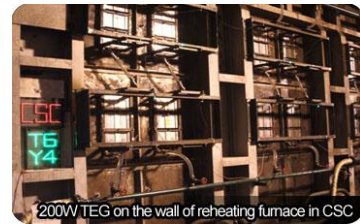
Figure 1-19: TEG used in China Steel Corporation (CSC) reheating furnace wall [26]
